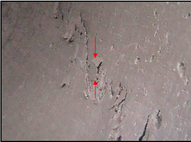
Figure 18. Spalling of concrete on inner wall of Specimen 3, along the shear crack.
