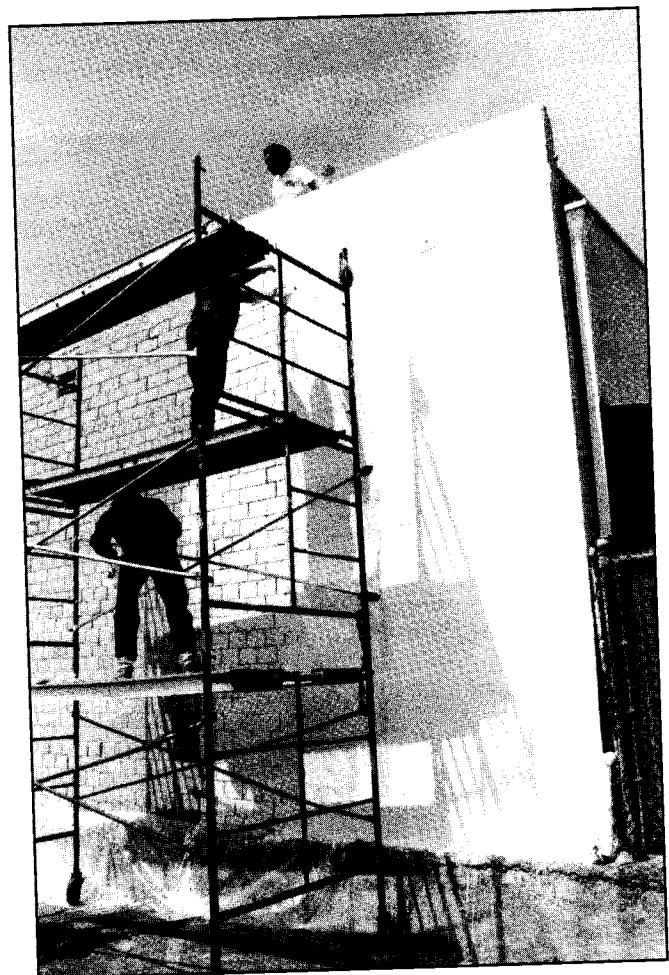
Fig. 12—Application of QuakeWrap ™ to the wall (Photo courtesy of External Reinforcement, Inc.)
