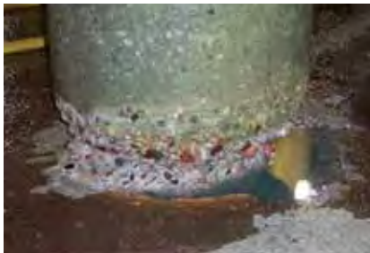
Effects of SX-EW electrolyte leakage on cell house concrete support columns.
