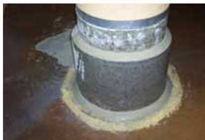
The traditional method of repairing damaged columns involved removing damaged concrete and rebar (top), inserting new rebar (center), and encapsulating the repaired column in a poured shell of polymer concrete.
